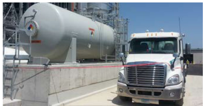
High-visibility magnetic level indicator with magnetostrictive transmitter supports the offloading of ammonia at a combined cycle power plant
