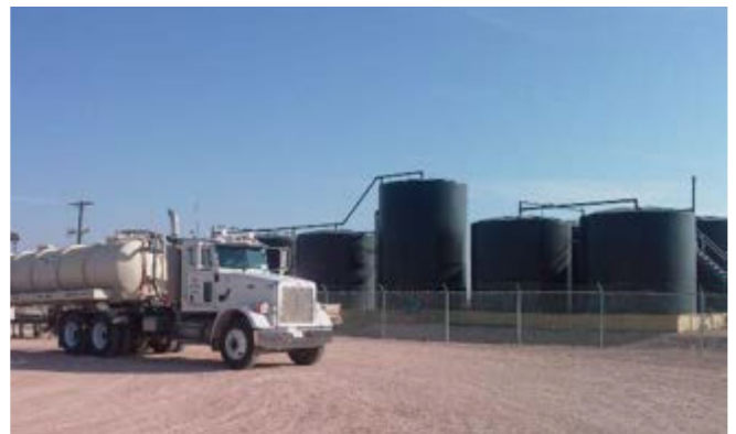
Figure 7: Truck unloading into tank battery for salt water / oil storage and separation
