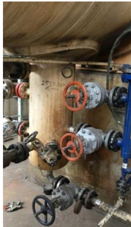
Figure 9: Boot for separation in a refinery (GWR transmitter installed in blue chamber at right)
