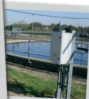
Vertical unistrut mounting near settlement tank
