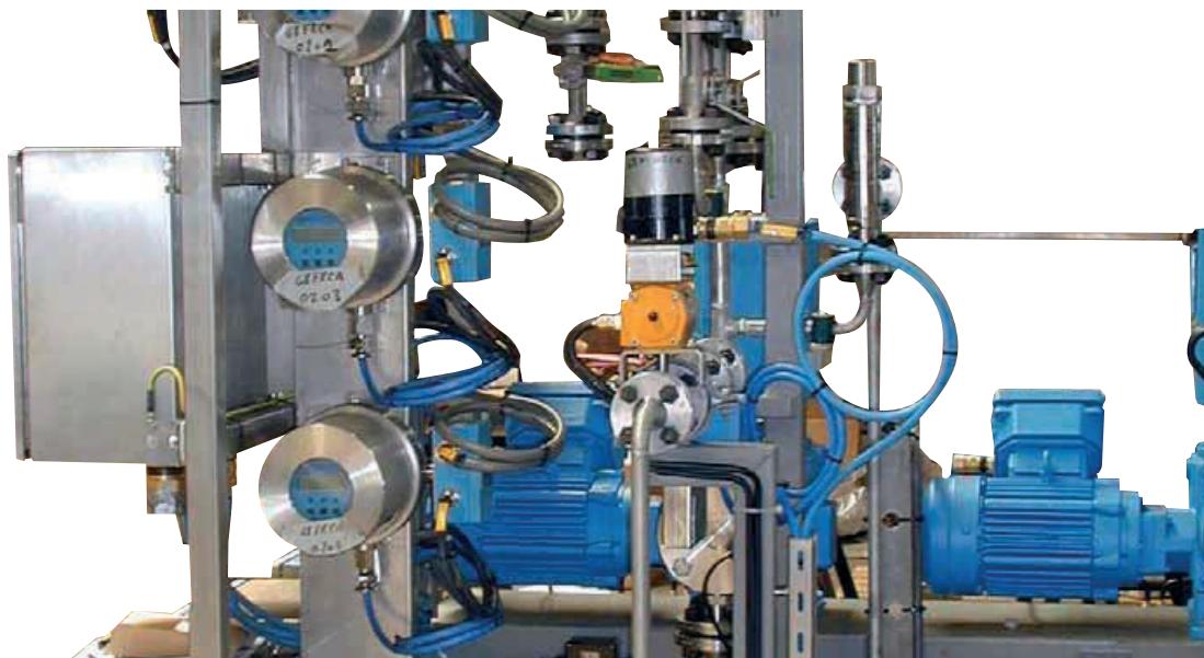
Oil & gas flow metering skid
